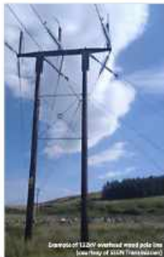
Example of 132kV overhead wood pole line (see list of 2024 restrictions)
